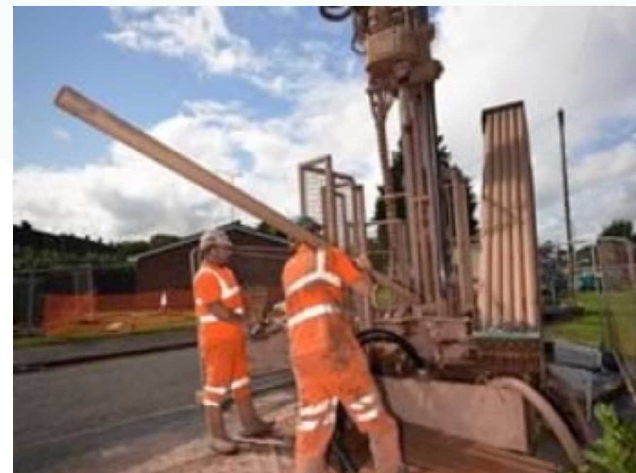
Pilot ground source heat pump project
