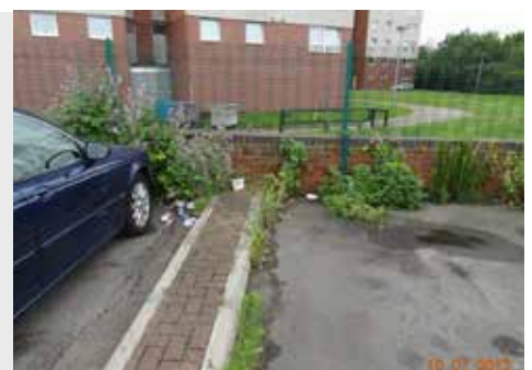
Grade D - Very poor
