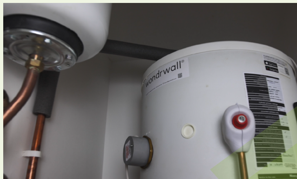
The Wondrwall heating system.
